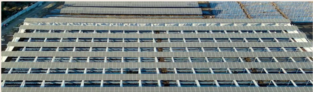
Figure 1: top view of ground mounted PV
