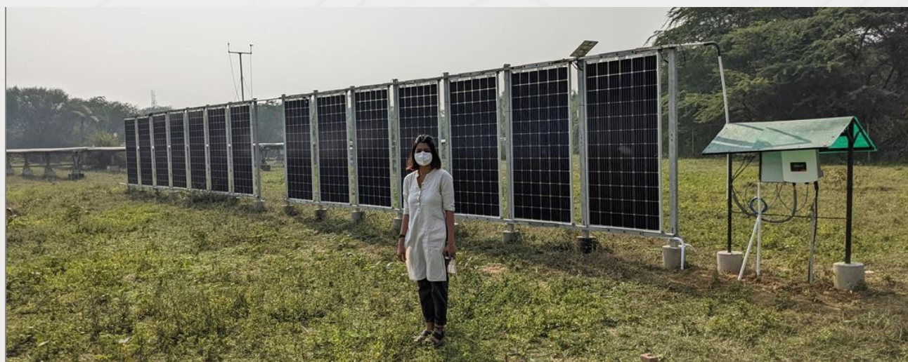
Figure 75. Vertical PV installation with bifacial modules at NISE (Credit: NSEFI)
