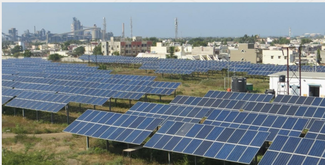
Figure 30. Panel view Gujarat State Electricity Company Limited- 1MW- Jamnagar
