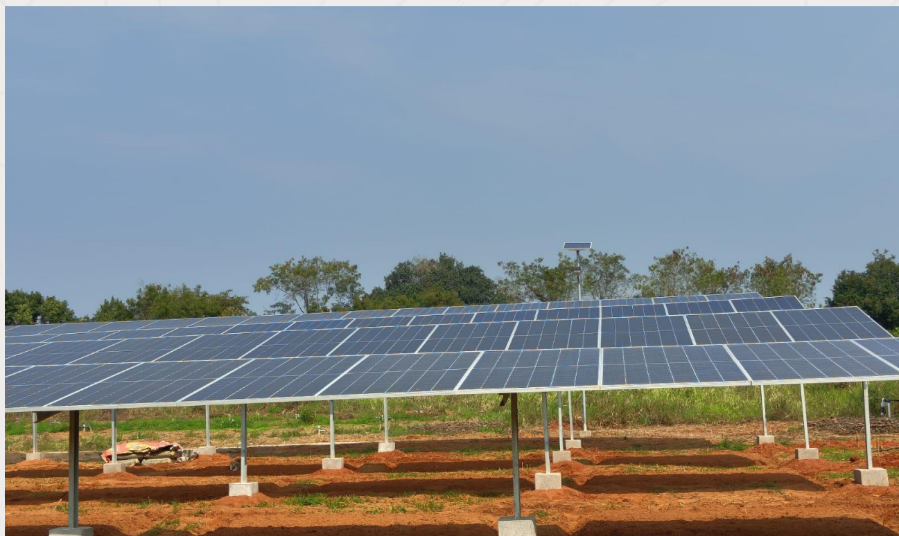
Figure 58. Panel structures of the 40Kwp plant of Odisha University of Agriculture and Technology
