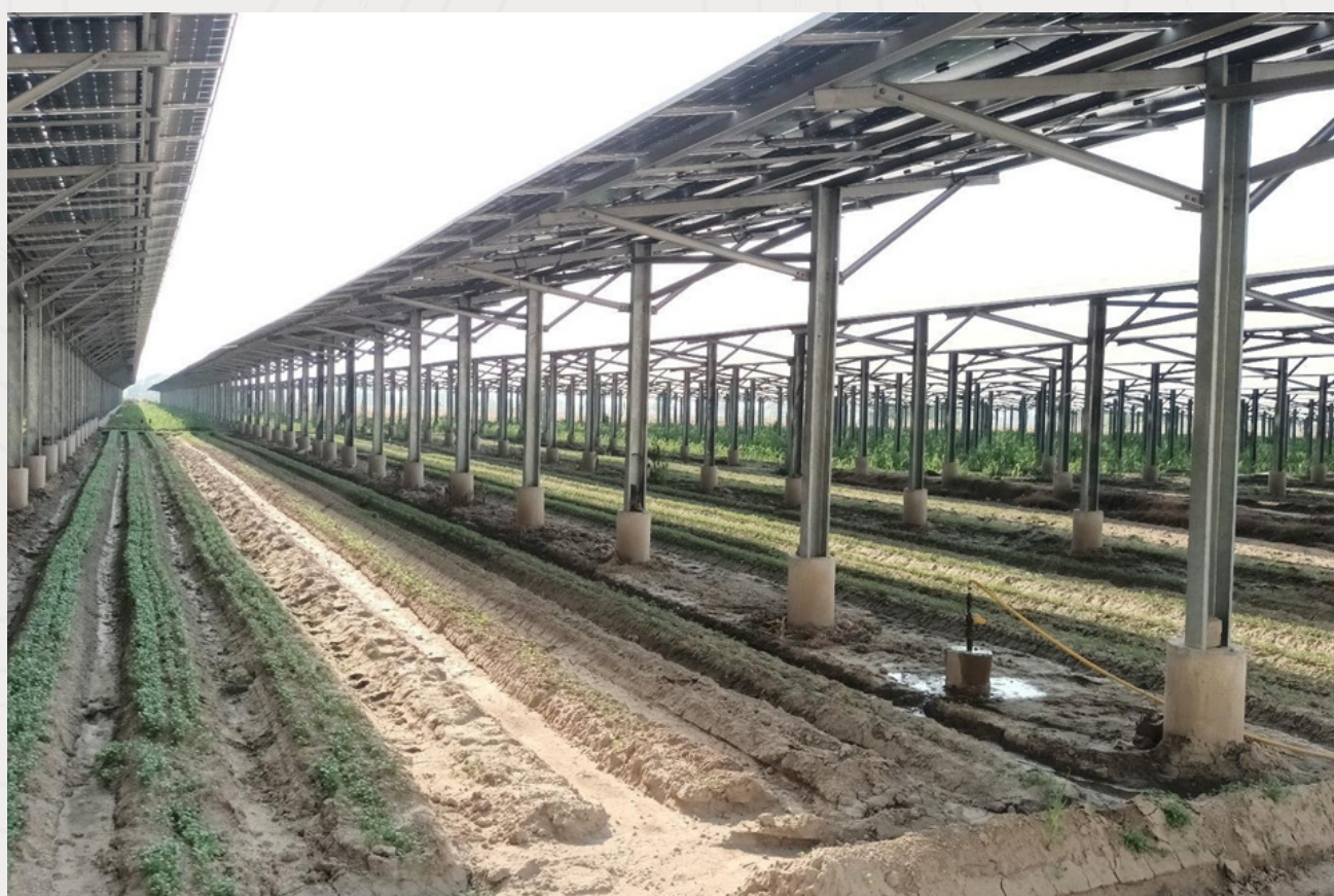
Figure 4. Panel structures of the 4.2 MW plant by Talf Solar
