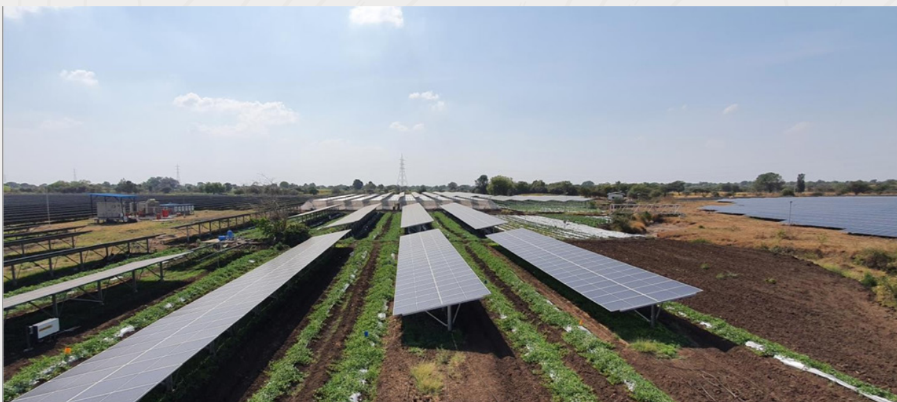
Figure 19. Section IV (Interspace) at Agrivoltaics plant near Parbhani (Credit: GIZ)
