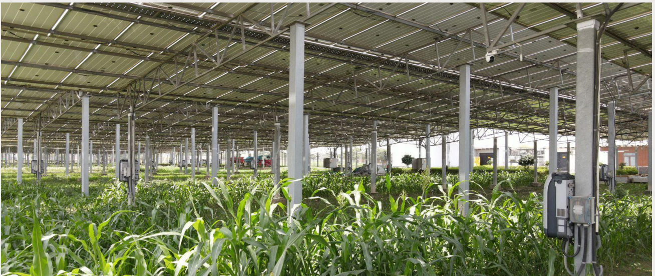
Figure 10. Panel Structure at the Sunmaster Agri PV Plant Issapur Dhasa 2 - 2.5 MW
