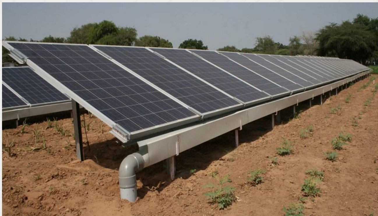
Figure 55. Agrivoltaics system with rain gutter at CAZRI (Credit: CAZRI)
