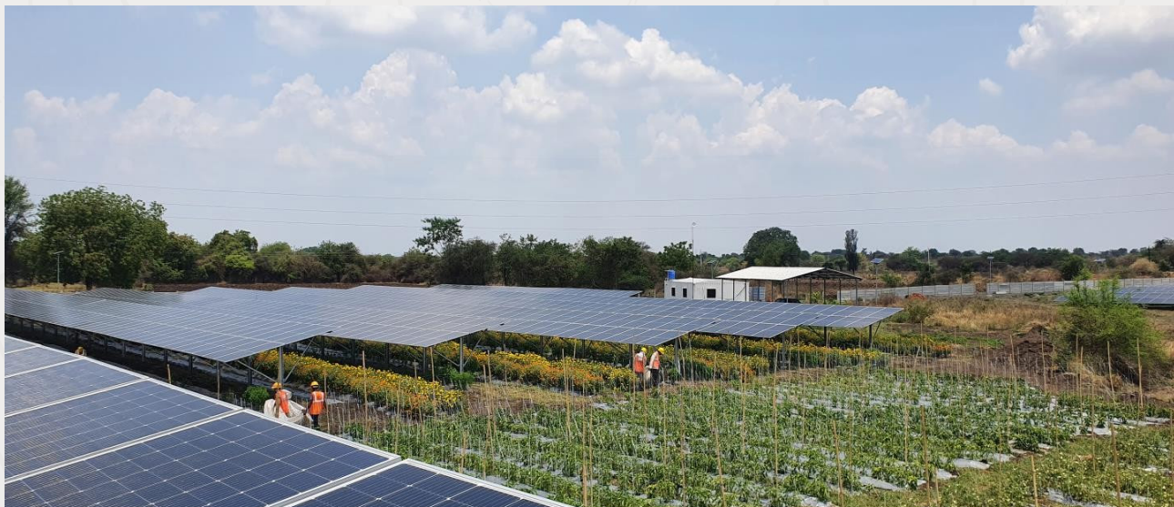
Figure 18. Overview of Agrivoltaics plant near Parbhani. (Credit: GIZ)
