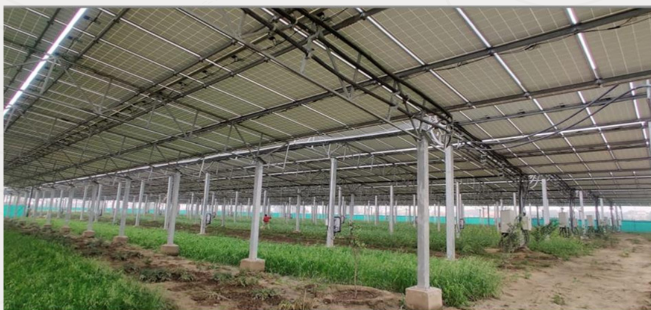
Figure 8. Below Panel View of SunMaster APV plant, Delhi (Credit: SunMaster
