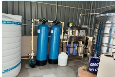
Power to RO Plant
