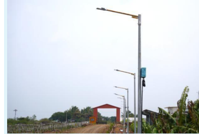
Power to Street Light
