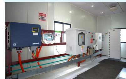
Modular Energy Storage System
